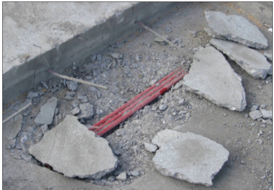
This small blowout is a result of a localized low point in the tendons between two higher points. Note the gap beneath the tendons and the slab, indicating how much the tendons lifted.
