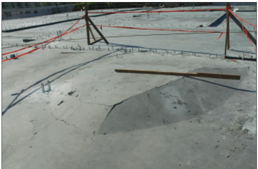
Top: Post-tensioning tendons are draped within the slab cross section. Bottom: Significant over-balancing of the weight of the concrete with post-tensioning can actually lift and crack the slab.
